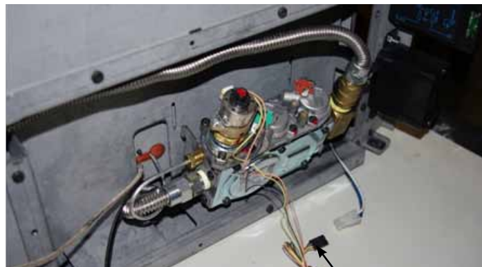
Cable from motor
